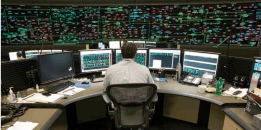
Fig. 17.20 Control center operators monitor the flow of electricity
