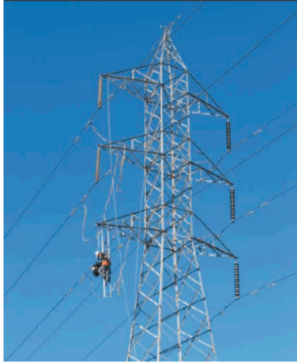
Fig. 17.5 High voltage transmission lines. (Courtesy of STAV Publishing)
