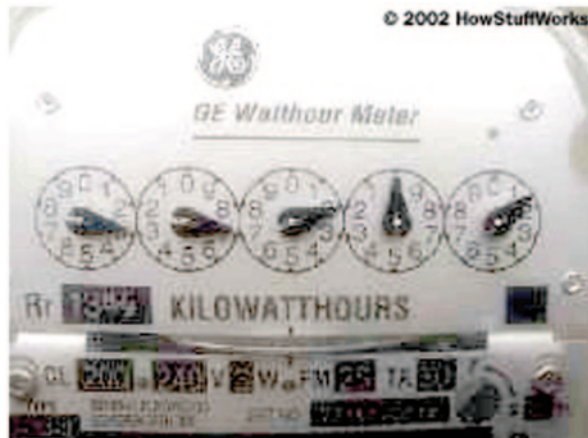
Fig. 17.16 Typical power meter. (Courtesy of PG&E)
